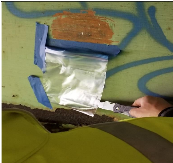
Lead Paint Visible
