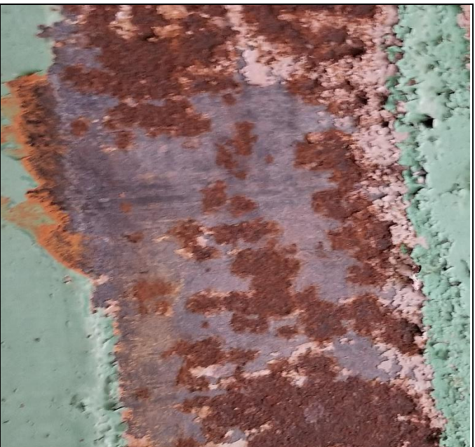
Appears to be original paint system, due to mil scale being present.
