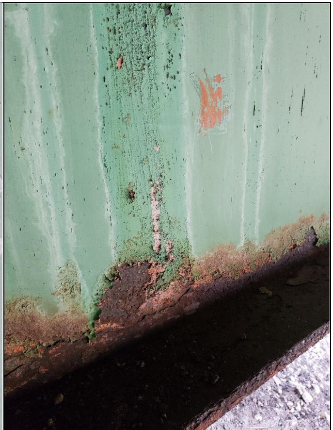
Flaking paint on bridge beam
