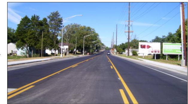
Clime Road Widening and Reconstruction, west of Harrisburg Pike, completed in October 2010
